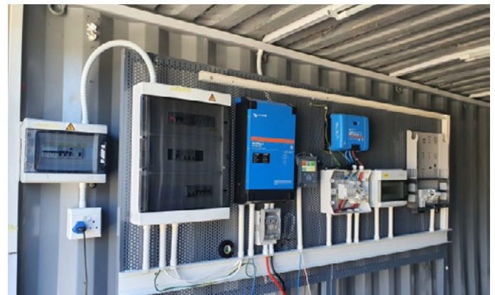
Work with real installations and PV systems set up at the academy
